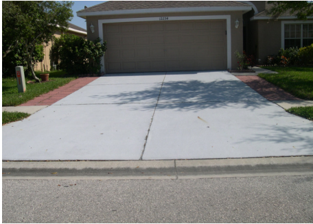
Unacceptable blue stain on driveway
