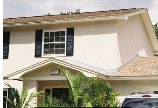
Unacceptable: unpainted flashing and roof drip edge
